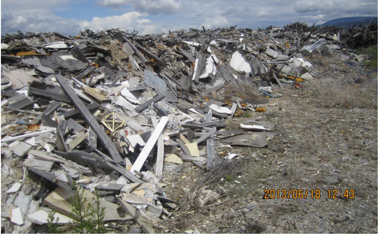
Photo 1. Unsorted Demolition Debris
