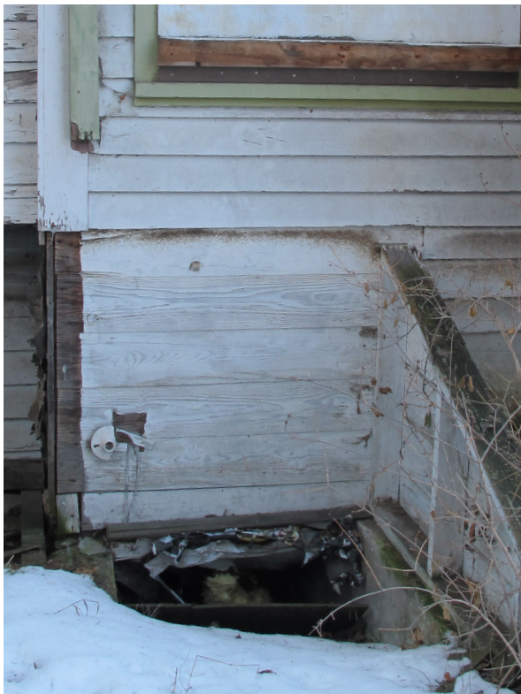
Portion of rear elevation showing opening to unoccupied partial basement, with exposed cast-in-place concrete foundation walls.
