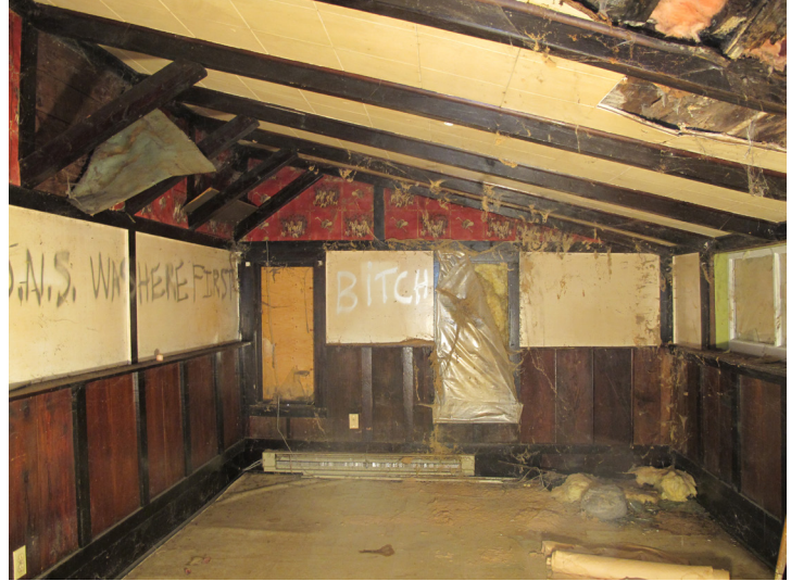
Interior space of the dining room (east early addition) showing exposed shed roof rafters with angle web wood members.
