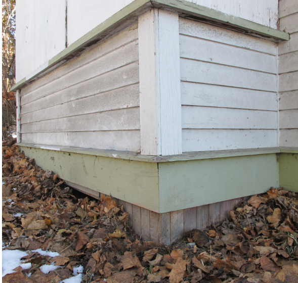
Lower portion of bay window at north elevation, showing wood lapped siding, window sill, and board trims. Note that foundation wall is clad in later vertical siding.
