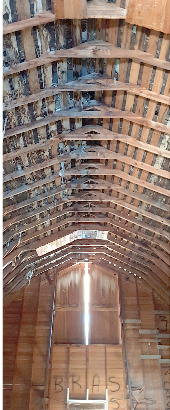
Photo showing interior side of the exterior wood-frame walls, looking north, and underside of the gambrel roof structure of the Surtees Barn.
