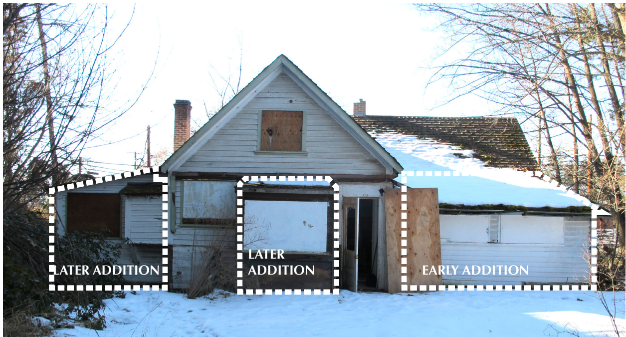
Perspectival view of the Surtees House showing partial east (rear) and north elevations (top); Rear elevation of surtees House to the east (bottom)
