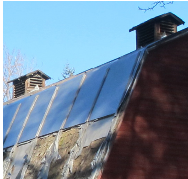
Photo showing typical deteriorated condition of two, existing monitor vents along the roof ridge.
