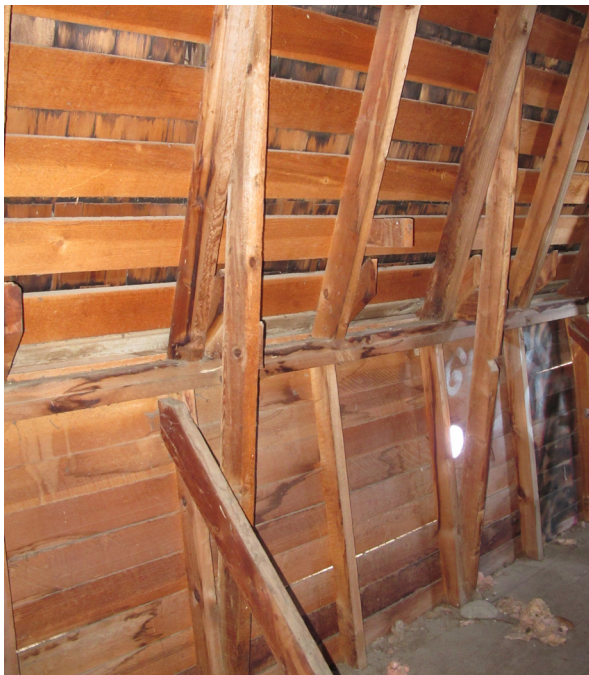
Interior side of the wall-to-roof interface, showing typical existing condition of the original wood materials.
