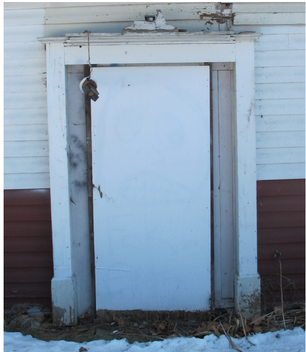
Photos showing original, existing door assembly at west return of south elevation (top), and later door surround trim at east elevation (bottom).
