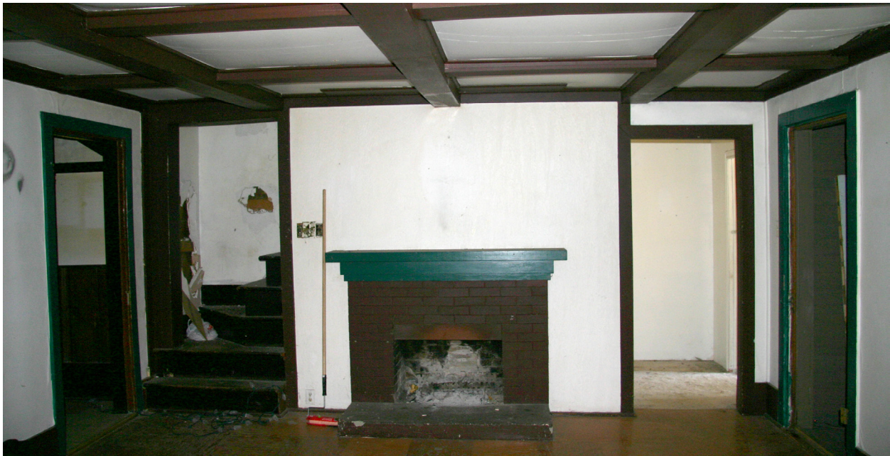
Photos showing surviving interior character-defining elements of Surtees House, including narrow winder staircase; brick masonry fireplace with raised concrete hearth and wood mantel; low ceiling with expressed horizontal beams and coffered-effect.
