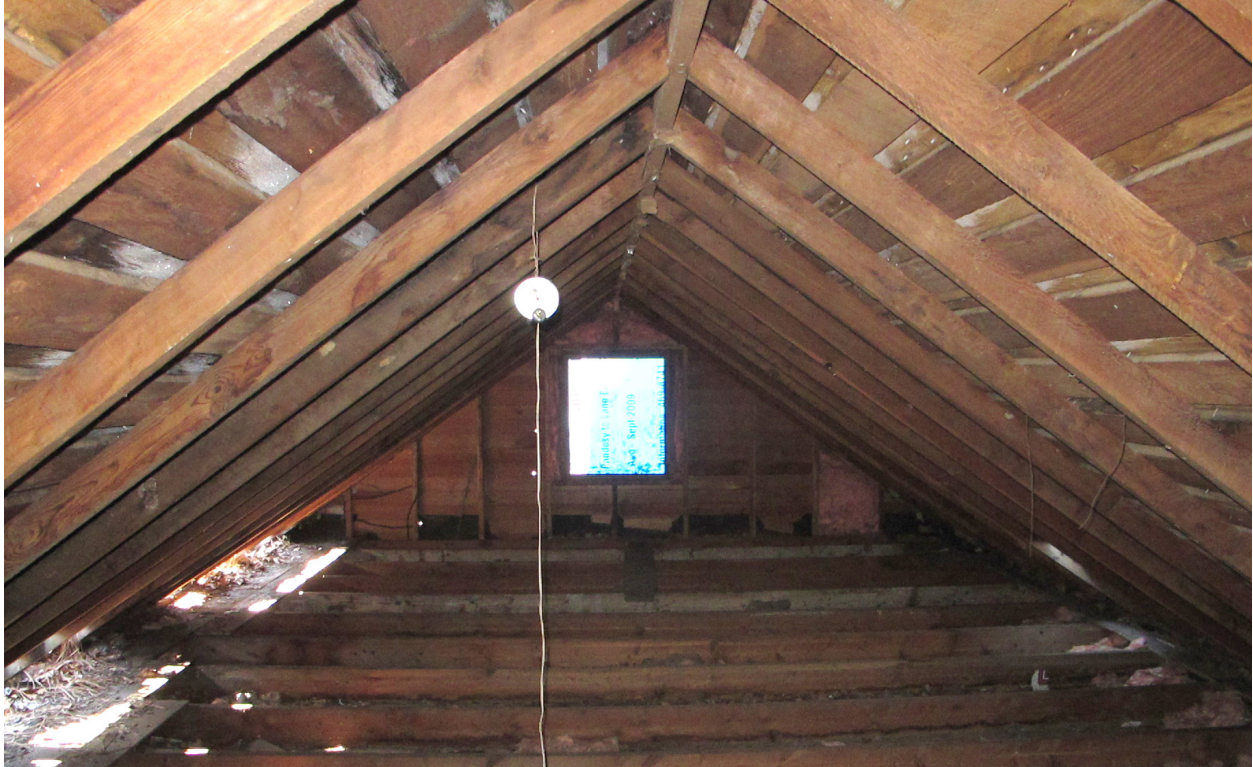
Photos showing side-gabled roof structure of the Surtees Barn extension, from exterior (top) and interior (bottom) side.
