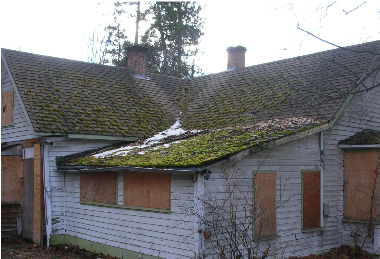
Existing condition of original, primary cross-gabled roof, with shed roof extension of early addition to the northeast portion of the house, as well as two original interior brick masonry chimney stacks along the roof ridges.
