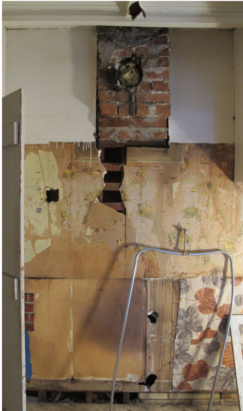
Interior brick masonry chimney flue terminating at midsection of the interior wall, partially showing wood structural support.
