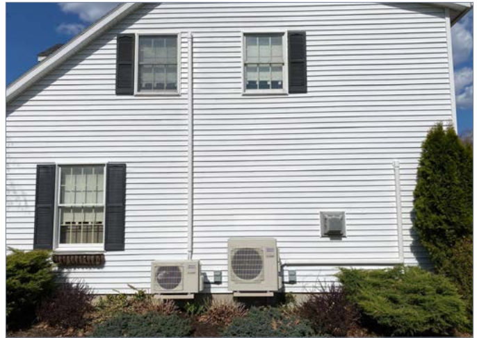
Figure 23: Upgrade mechanical systems to improve thermal performance. Install new, properly-sized electric heat pumps, boilers, hot water tanks, and energy-efficient appliances that meet Energy Star ratings or higher.
