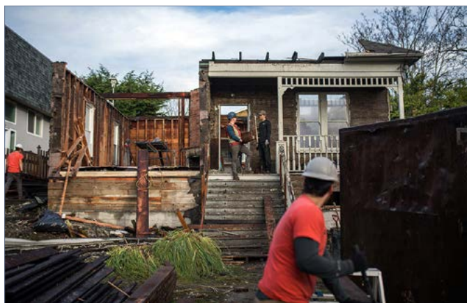
Figure 21: Deconstruct buildings instead of demolishing them to salvage materials for reuse and re-manufacturing.
