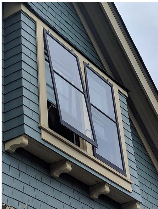
Figure 22: Achieve thermal efficiency by repairing and maintaining existing wooden windows. Installing wood-framed storm windows can further improve thermal efficiency and provide sound abatement.
