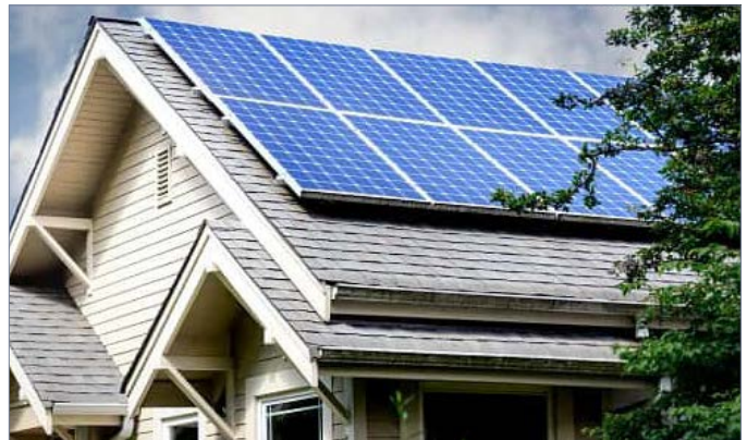
Figure 25: Place solar panel installations on building elevations, roof planes, or ground locations that respect the landscape and minimize visibility from the street.
