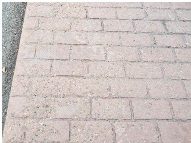
Figure 17: Salt damage along East pathway bordering asphalt parking area
