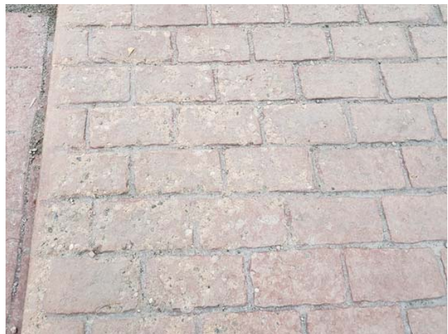
Figure 28: Salt damage along East side of plaza
