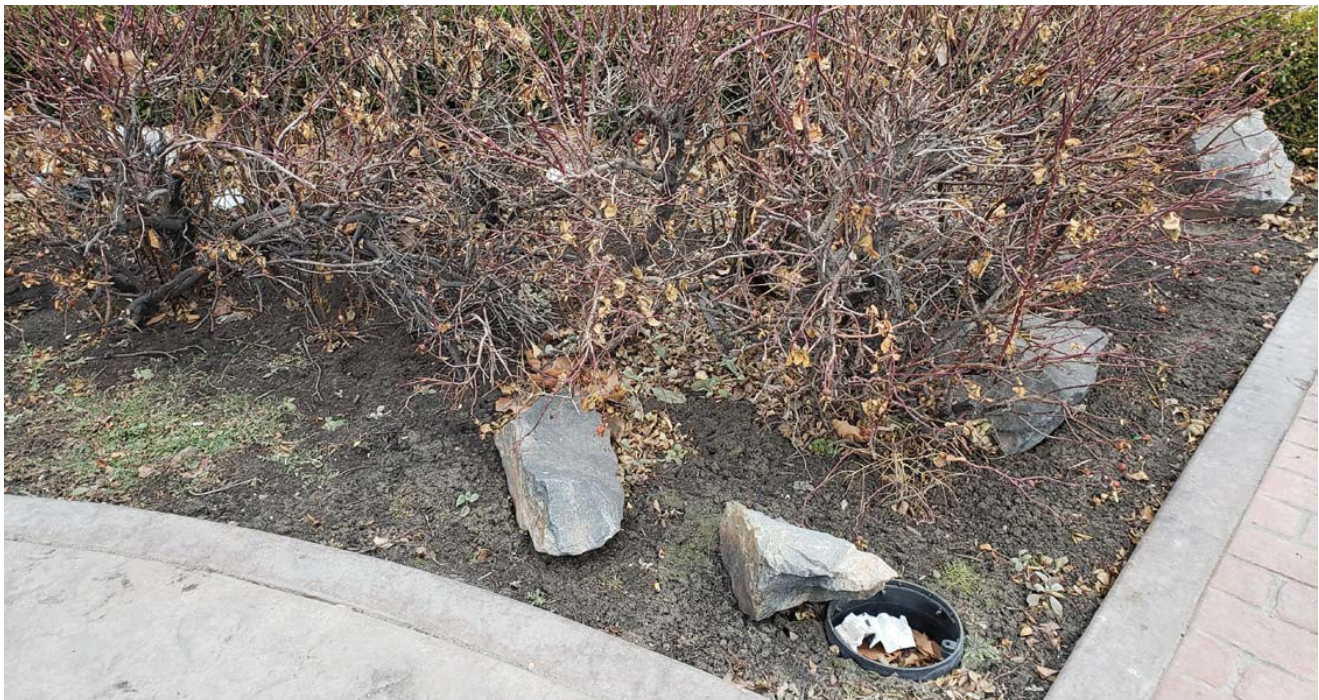
Figure 10: Irrigation valve box missing lid and garbage behind roses in North planting bed. Another valve box was missing a lid in the southwest planting bed.
