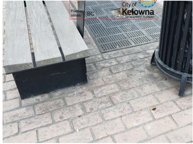
Figure 26: Darkening on stamped concrete paving
