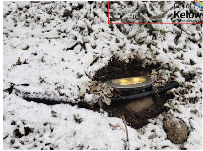
Figure 9: Exposed irrigation line visible in raised planter near upright.
