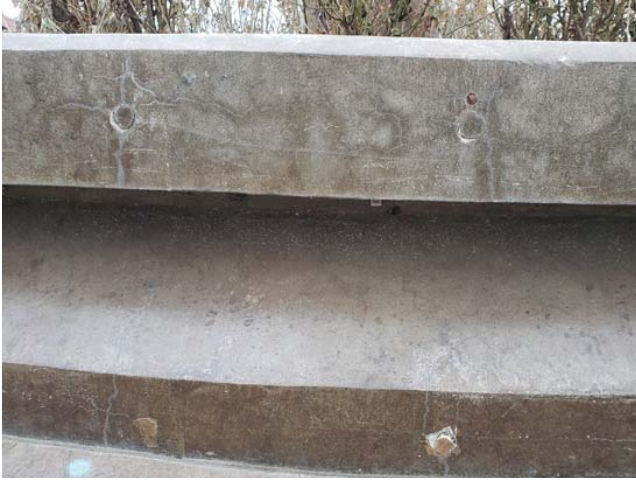
Figure 13: Additional cracking along wall of raised planter
