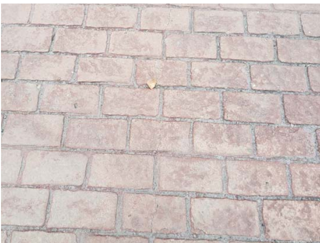
Figure 16: Small crack in surface of stamped concrete paving
