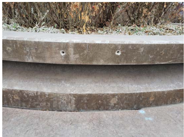
Figure 12: Holes in wall of raised planter
