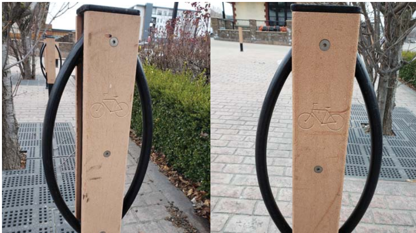
Figure 23: Scuffing and wear on bike rack posts
