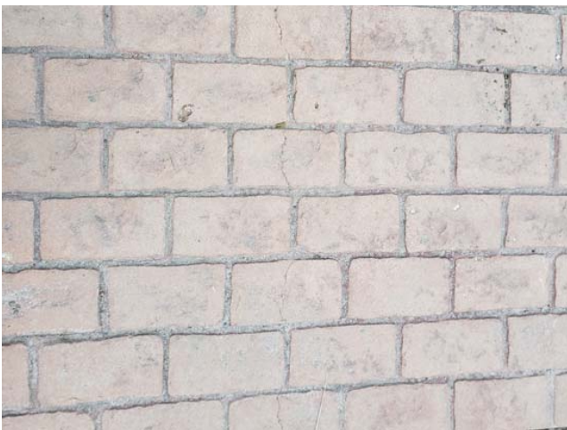
Figure 27: Small crack in surface of stamped concrete paving
