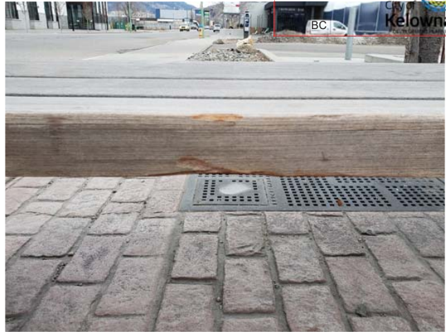
Figure 21: Chip damage on front of timber bench slat
