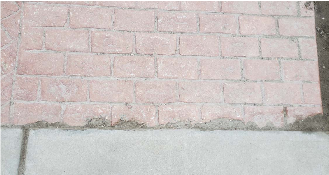
Figure 15: Cracking of stamped concrete paving along edge of municipal sidewalk at Southeast corner of garden, off Clement Avenue
