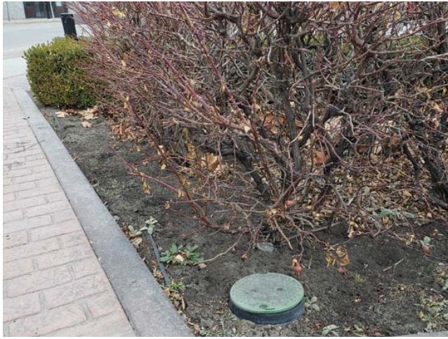
Figure 8: Exposed irrigation lines visible in planting bed at Northwest corner.
