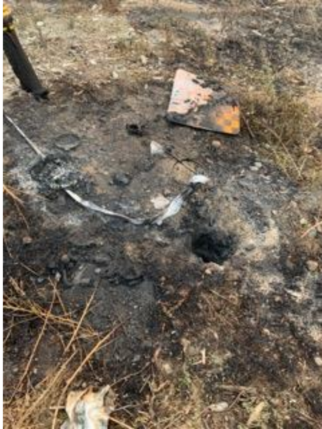
LATERAL CONNECTION BURNT
