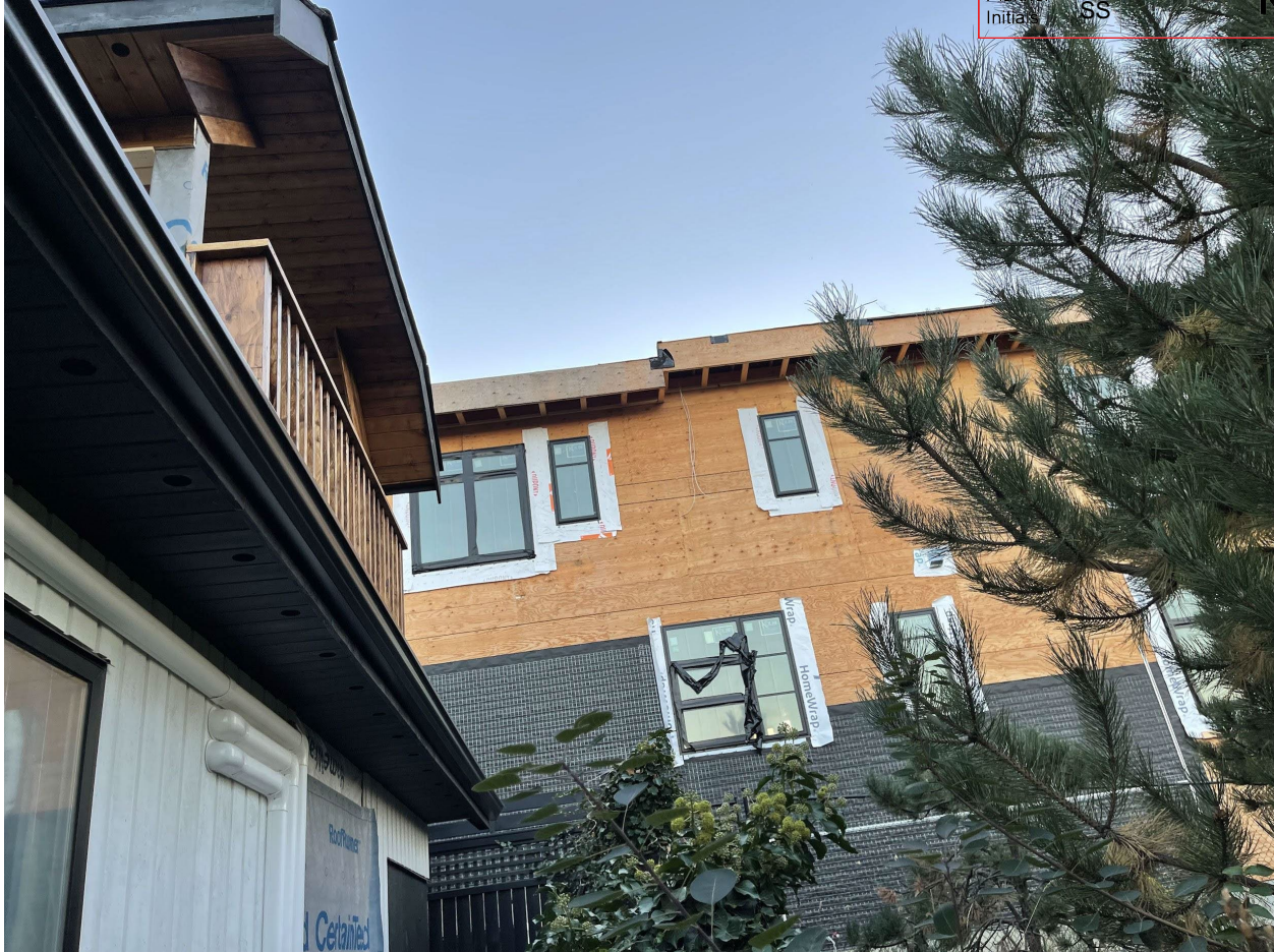
View from west side of accessory building towards the south to the new build
