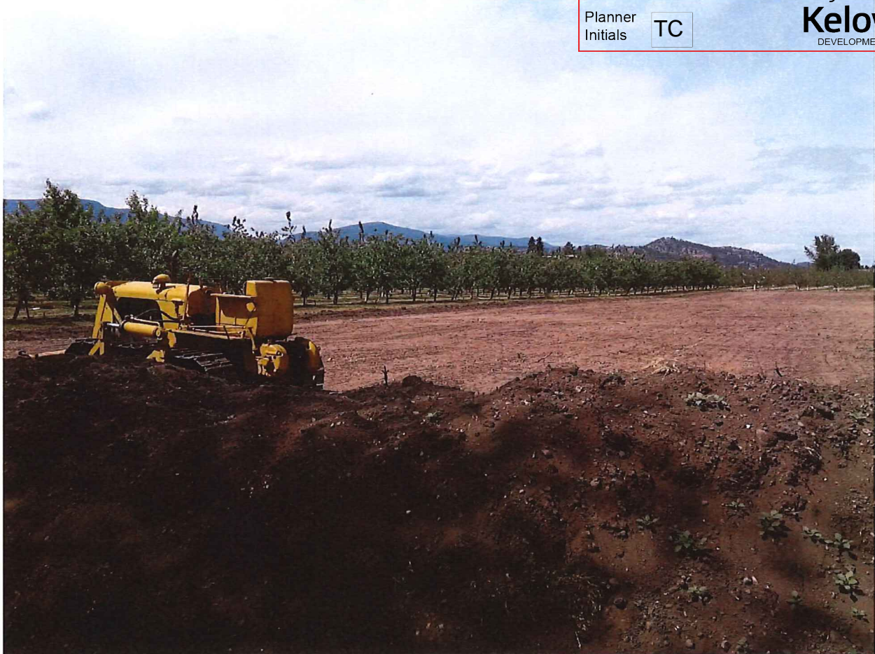
Photo 2: area in question looking North; note topsoil surrounding area remains in place. The scale shack will sit approximately where the Cat is now.
