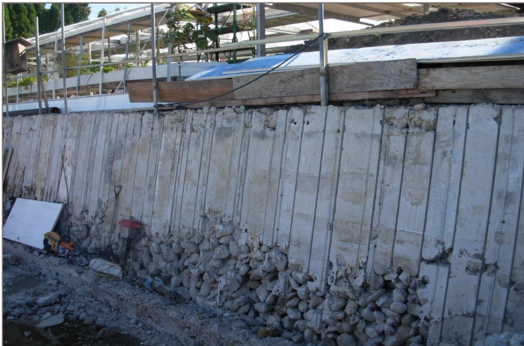
Photo 2: Upper wall center area. Gravel to boulder size rocks bound with mortar.
