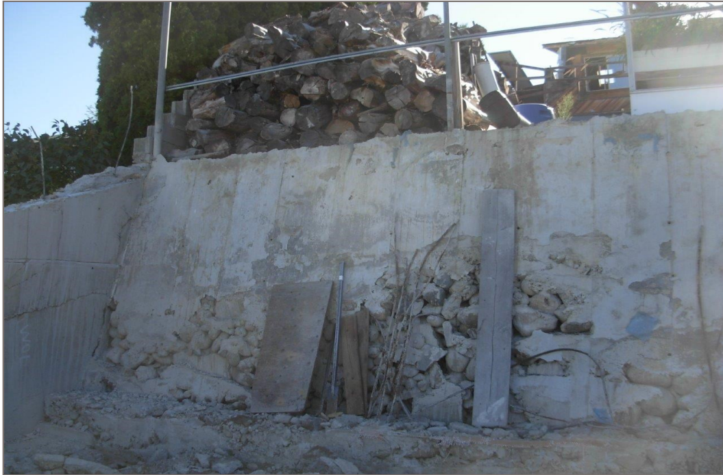
Photo 3: Upper wall north end. Coble to boulder size rocks bound with mortar.
