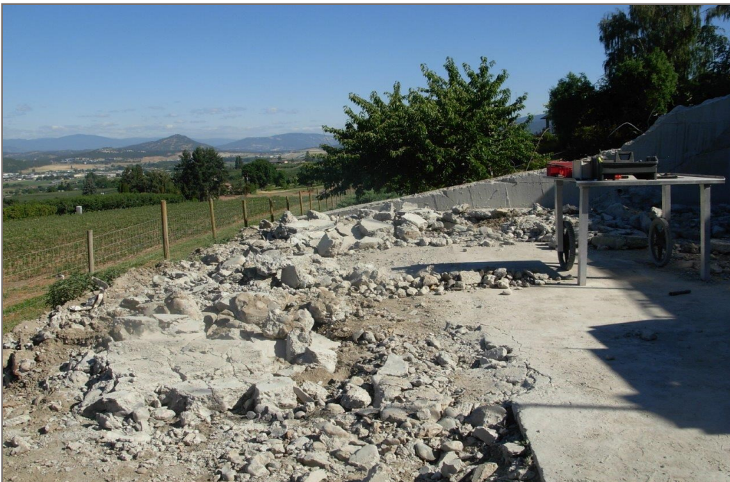
Photo 12: Surcharge flat area above steep backslope of lower wall.
