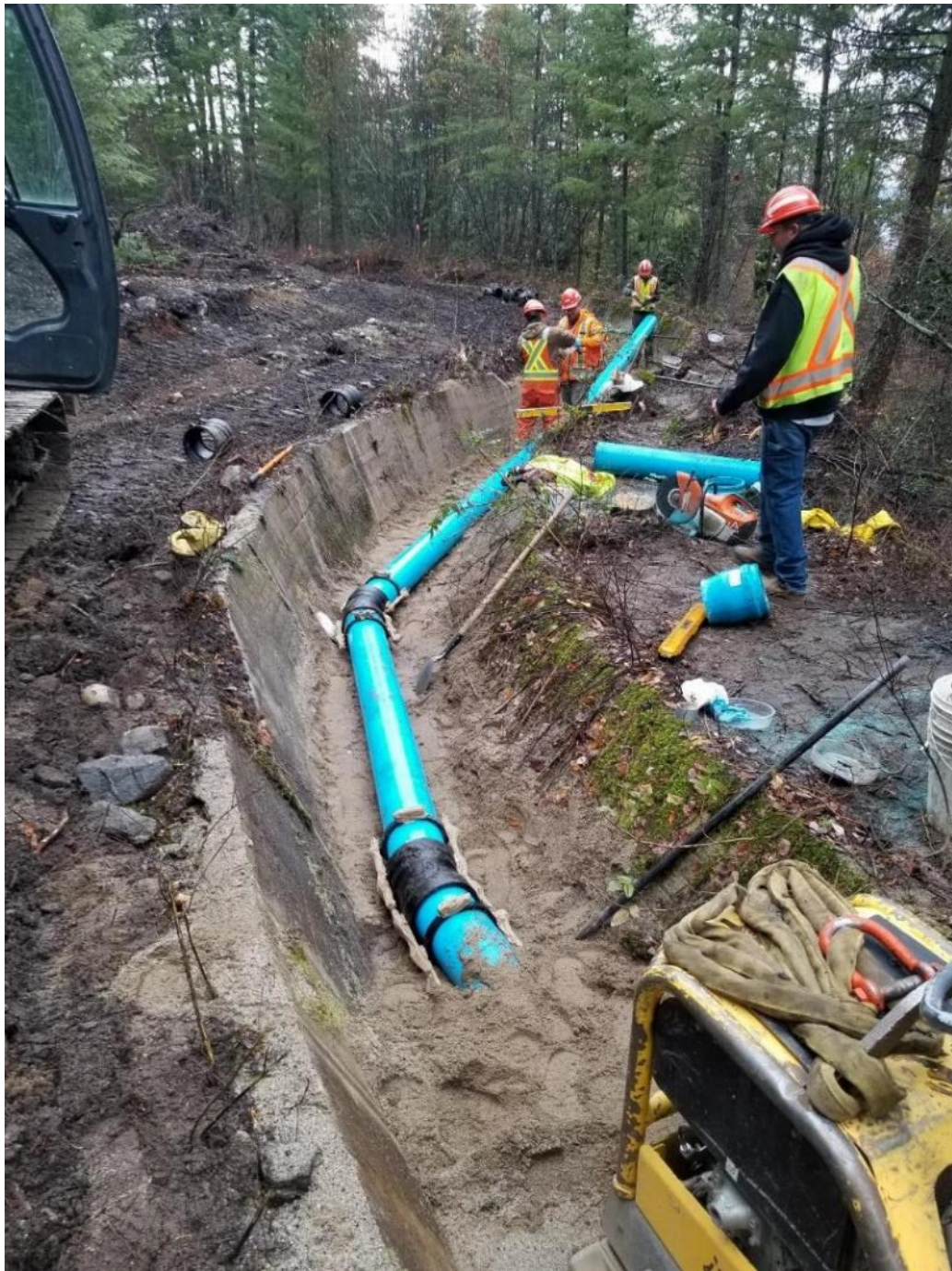
200mm watermain through Myra Bellevue Provincial Park. Alignment making use of abandoned irrigation flume
