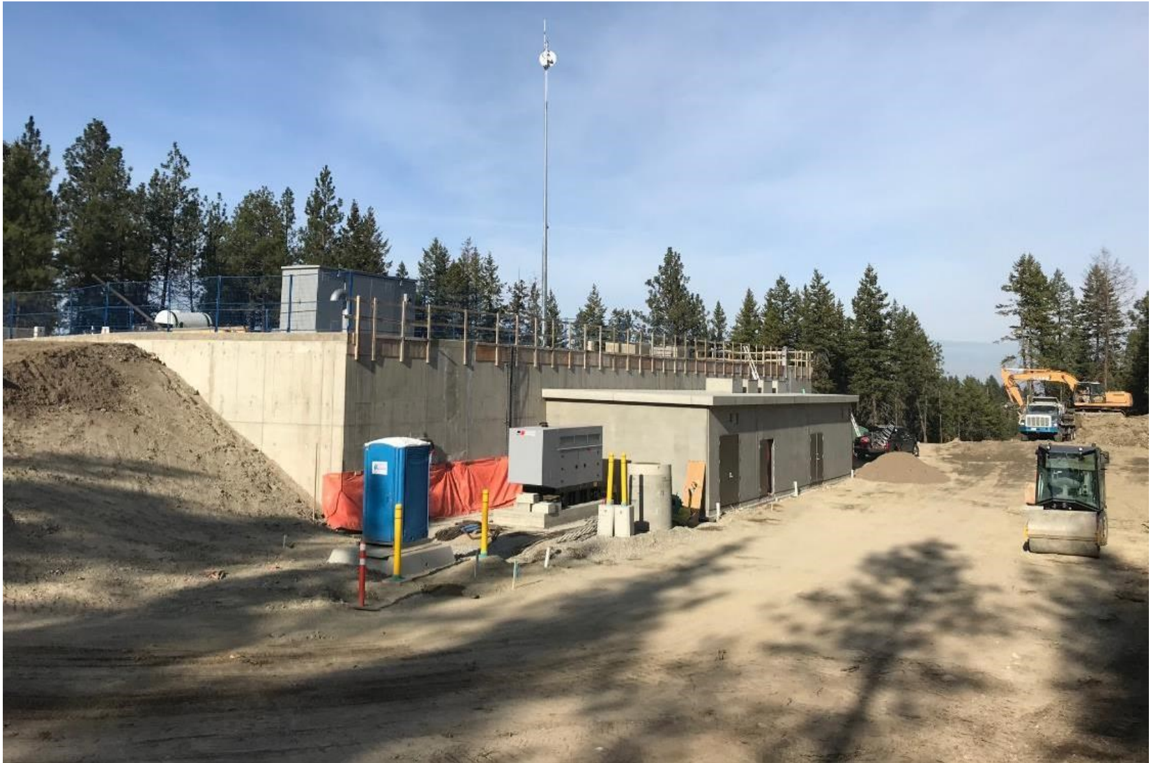
Jean Pump Station and Reservoir
