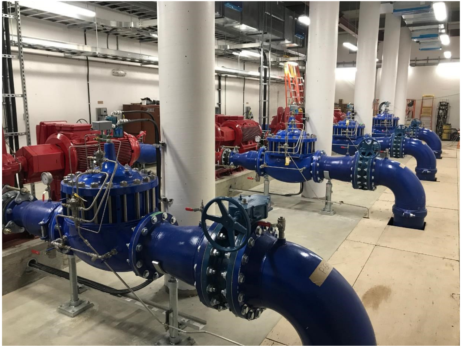
Stellar Pump Station
