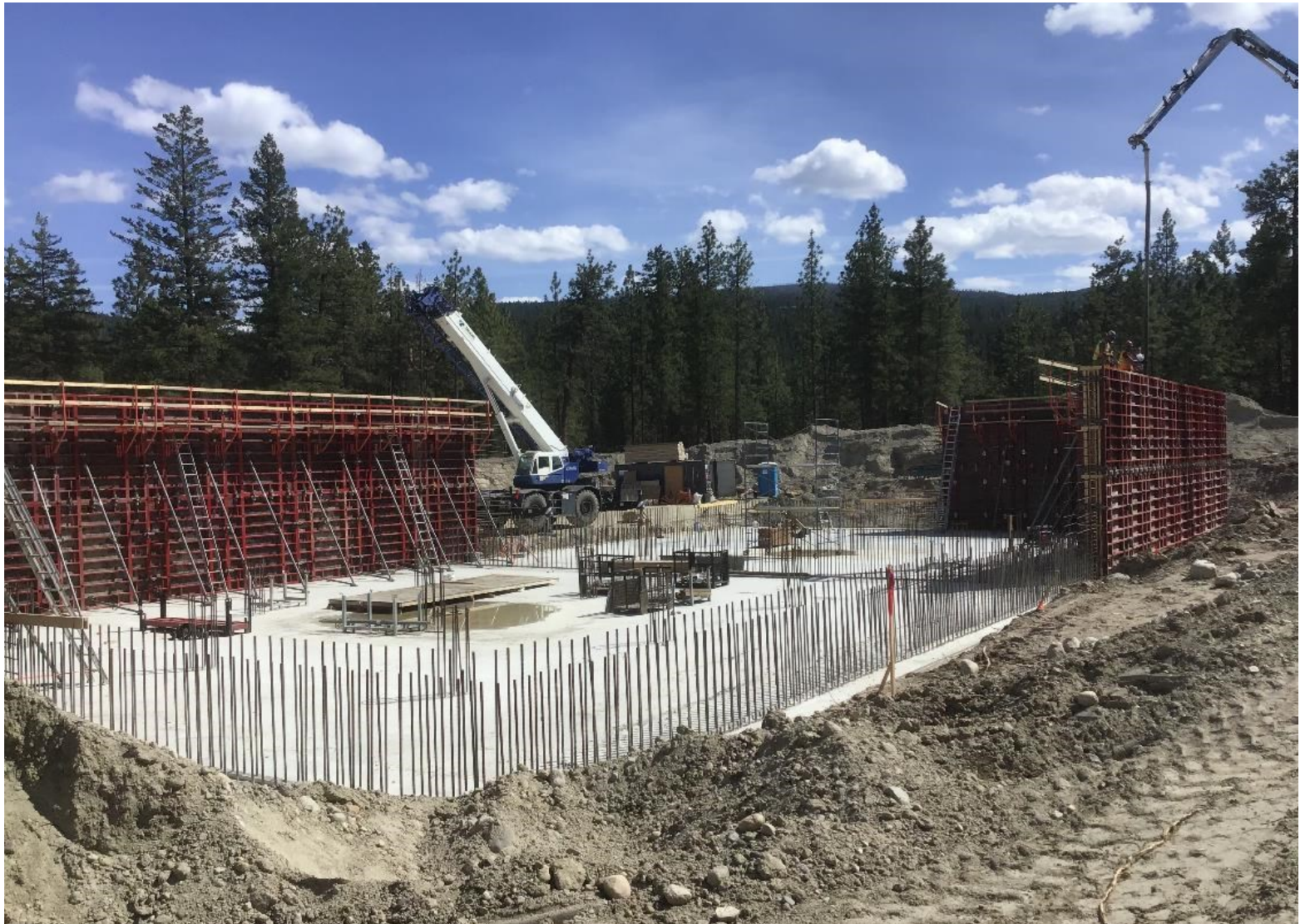
Jean Pump Station and Reservoir
