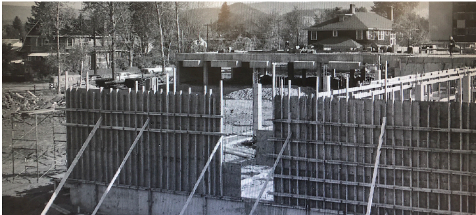
View of construction of the Strathcona building in 1969. The Cross House is visible to the left of the historic Nurses Home.
