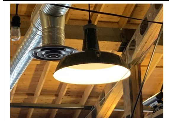
Re-wired light fixture – Laurel Packinghouse
