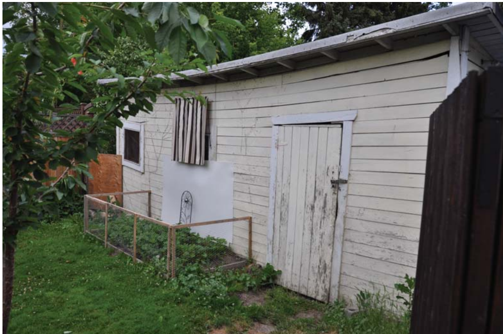
Photo 12. Dilapidated shed in northeast corner of property to be removed.
