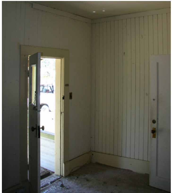
Surviving original v-joint panelling on walls and ceiling of front hall, showing original main entrance door to the left.
