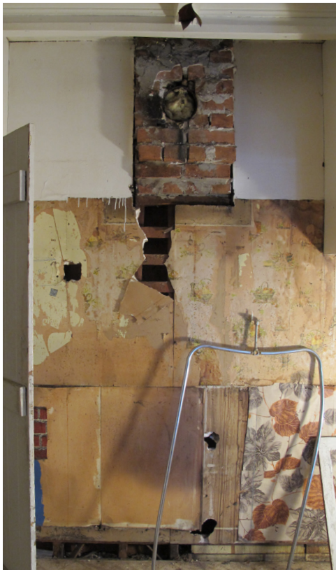
Interior brick masonry chimney flue terminating at midsection of the interior wall, partially showing wood structural support.
