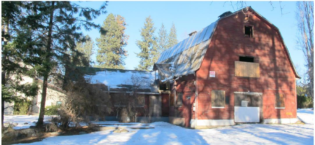
Archival photo showing south elevation of Surtees Barn with cross of church in the background (top; date unknown); photo showing existing condition of Surtees Barn, as viewed from southwest, with St. Andrew's Church in the background.
