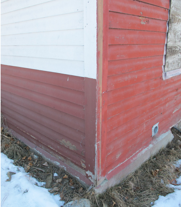
Northeast corner condition of the existing, original exterior walls of the Surtees Barn, showing unsympathetic paint finish.
