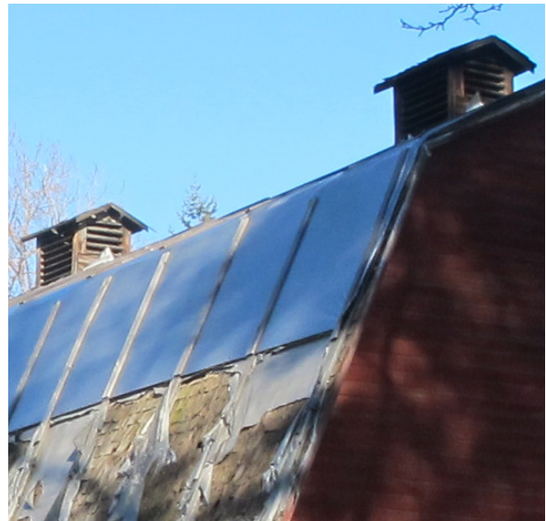
Photo showing typical deteriorated condition of two, existing monitor vents along the roof ridge.
