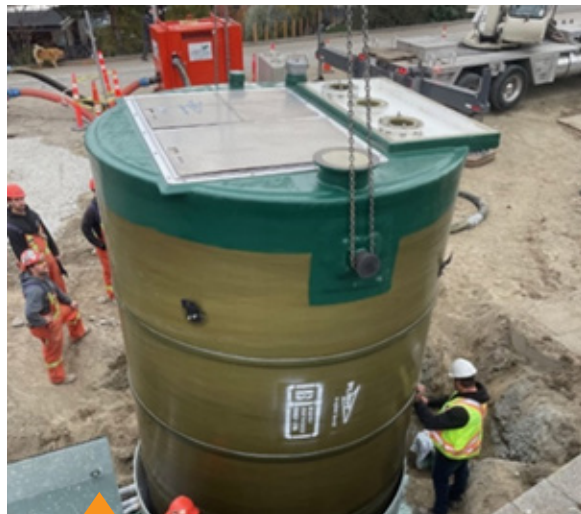
The City operates 44 lift stations, which transfer wastewater from a lower level to a higher level to transport it to the wastewater treatment plant.
