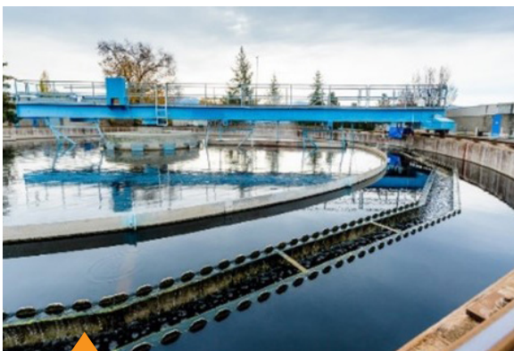
Before filtering and UV disinfection, wastewater goes through primary and secondary clarification, which removes solid waste and nutrients.
