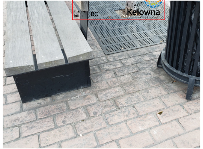
Figure 26: Darkening on stamped concrete paving
