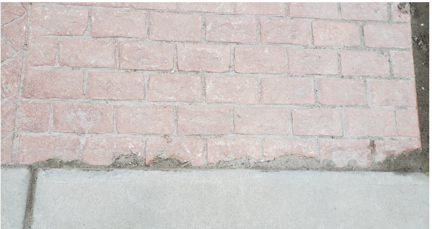
Figure 15: Cracking of stamped concrete paving along edge of municipal sidewalk at Southeast corner of garden, off Clement Avenue
