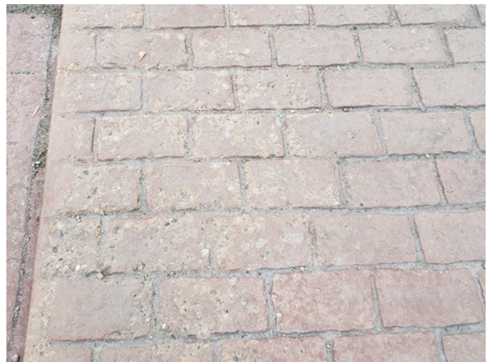
Figure 28: Salt damage along East side of plaza
