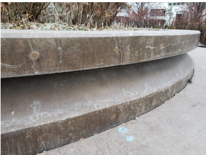
Figure 11: Cracking and scratches along top edge of raised planter
