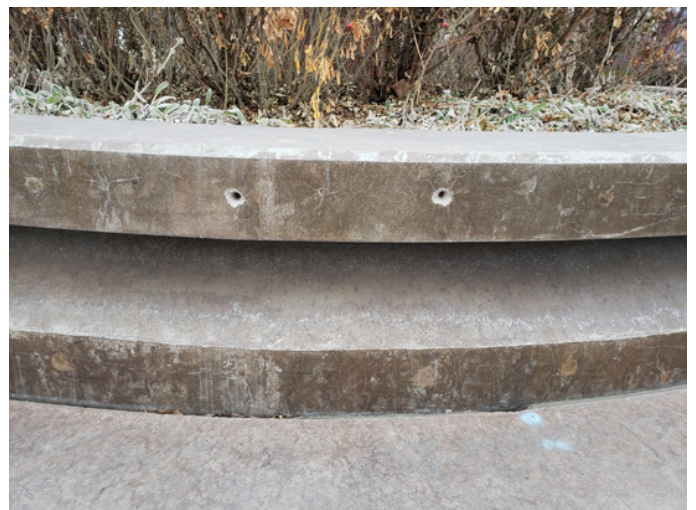
Figure 12: Holes in wall of raised planter
