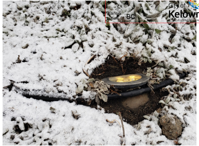
Figure 9: Exposed irrigation line visible in raised planter near uplight.
