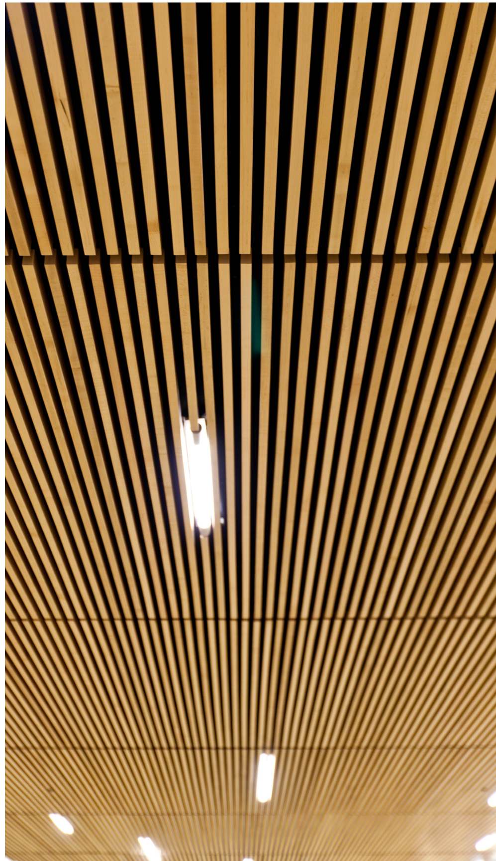
WOOD SLATTED CEILINGS
