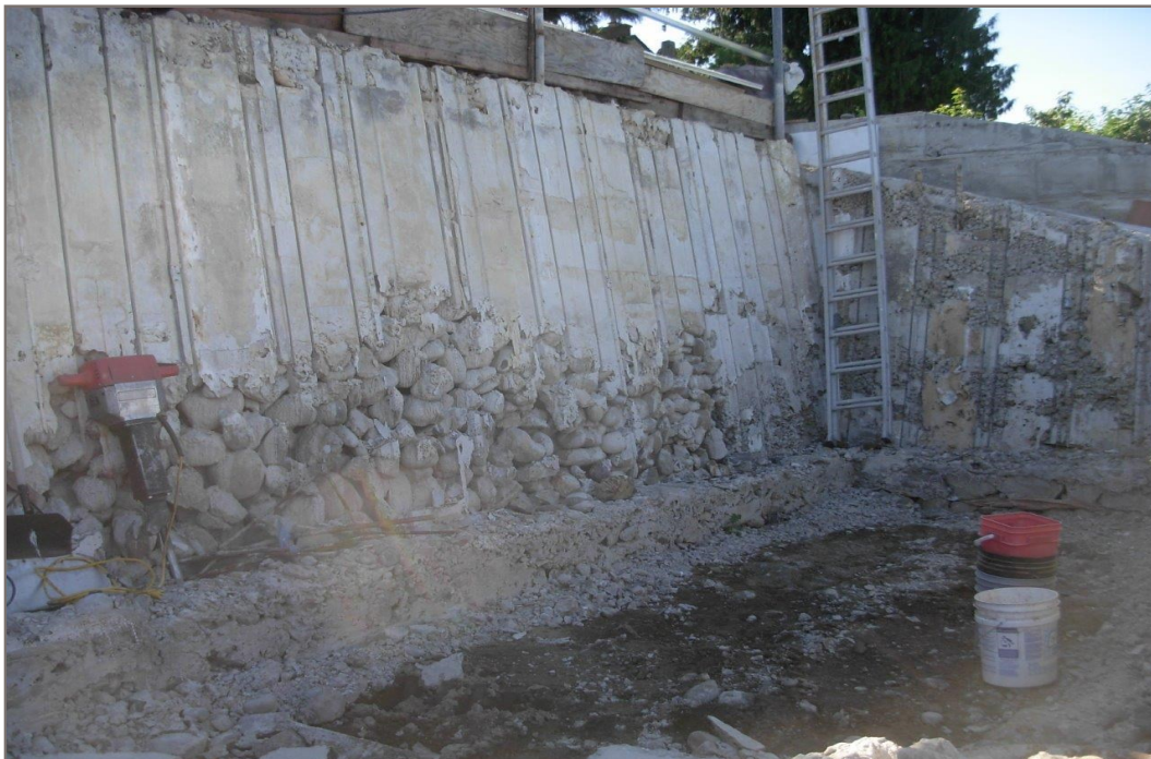
Photo 4: Upper wall south end approximately 2.6 m high. Cobble to boulder size rocks bound with mortar.
