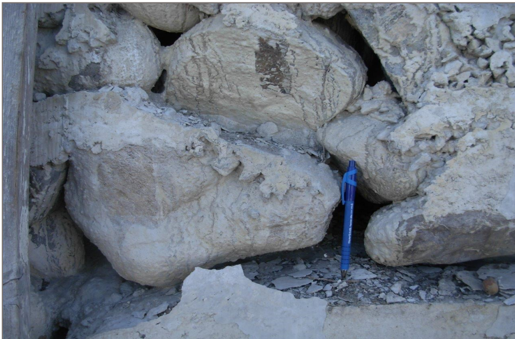
Photo 6: Upper wall cobble to boulder size rocks bounded with mortar. Significant voids shown.
