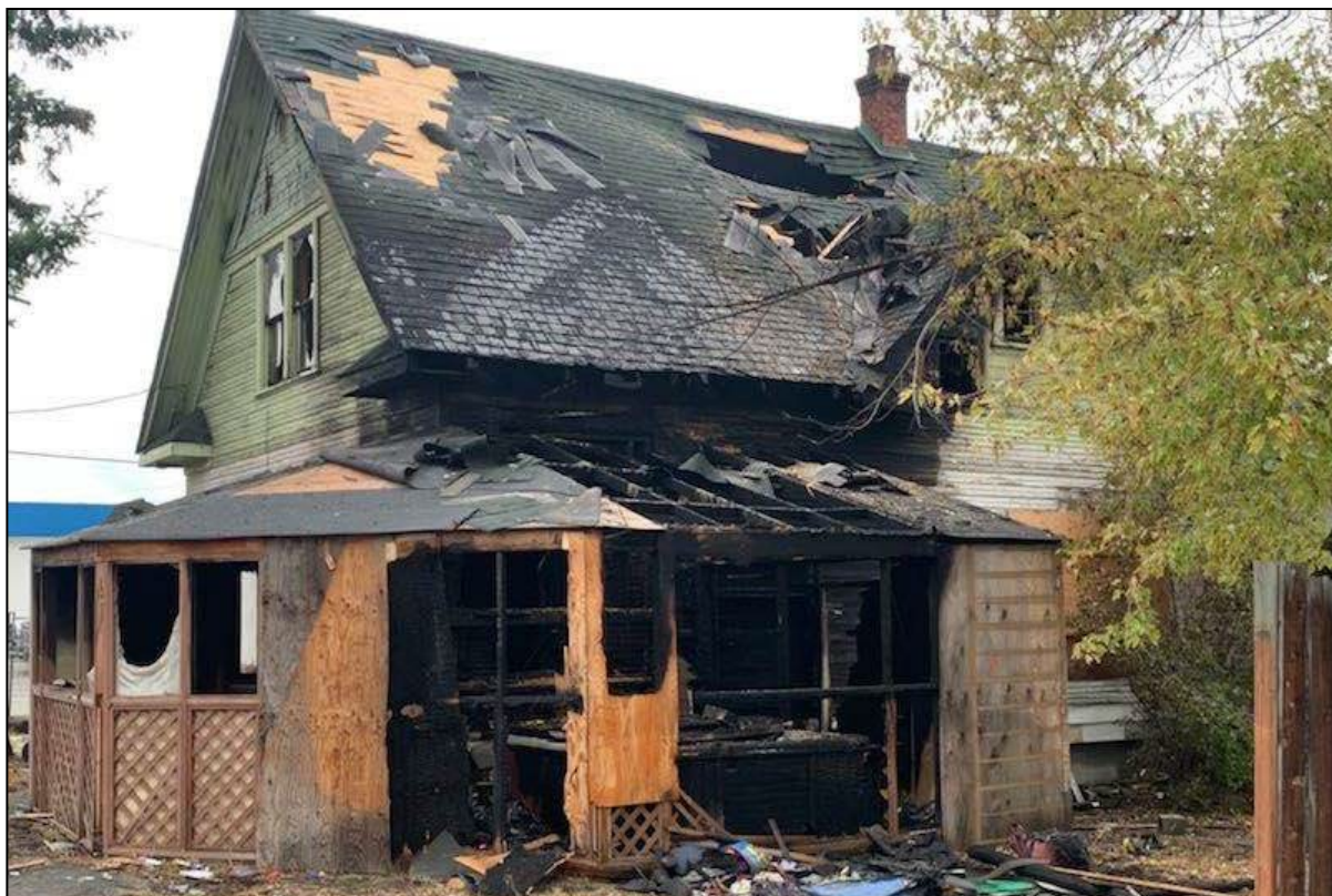
Fig. 1: Southeast corner view of 180 Hwy 33 E, illustrating some of the fire damage. (Source: An, 2020)
